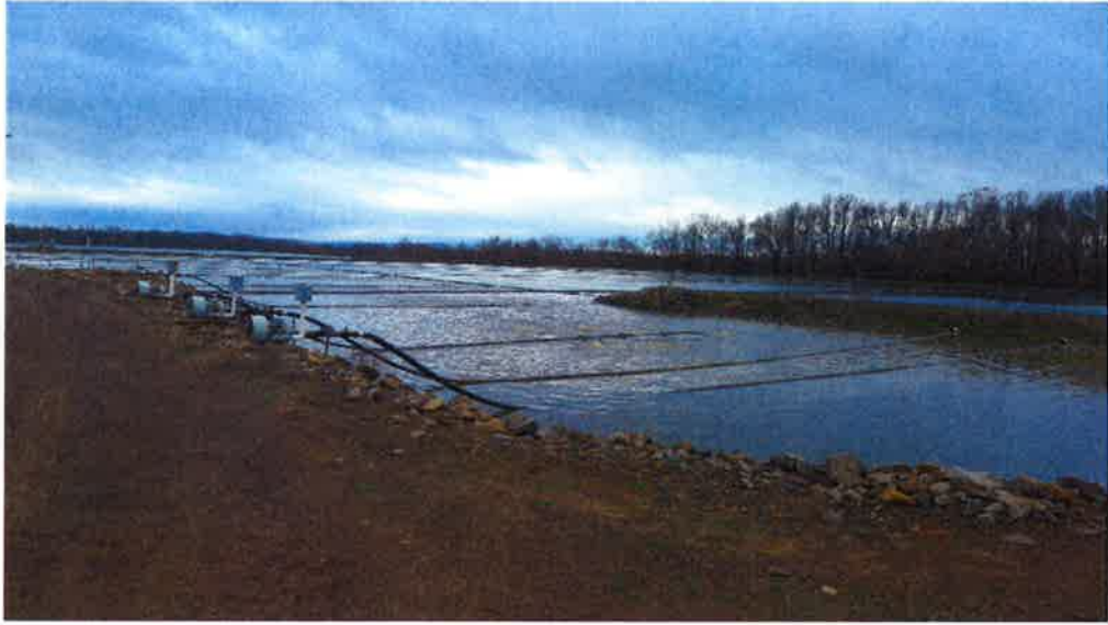
Aerators in Lagoon 1 Looking east
