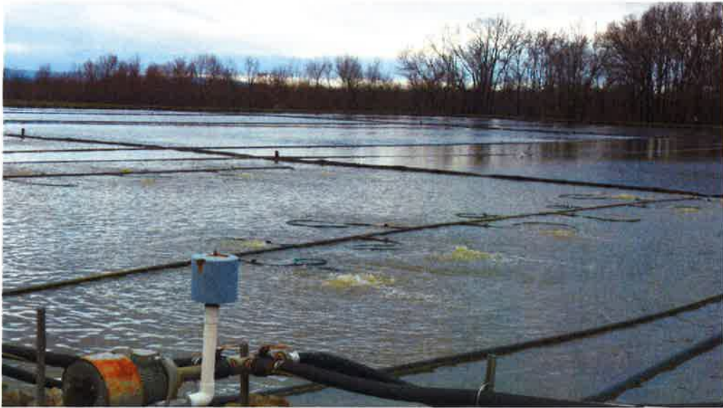
Aeration in Lagoon 1 Looking Southeast
